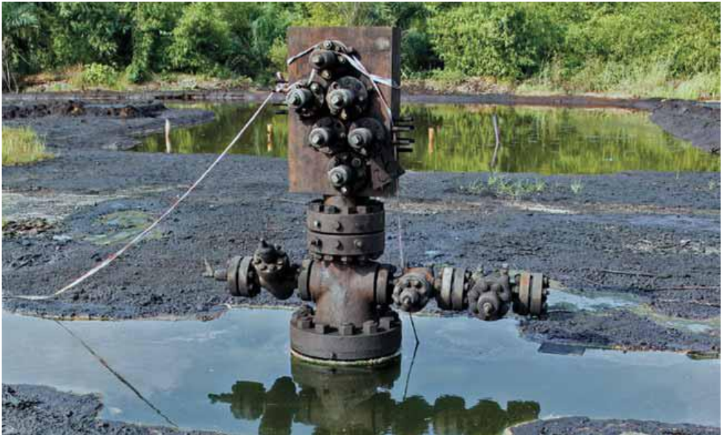
Plate 1: Abandoned Wellhead with Spill in Bomu (Source: UNEP, 2011)
